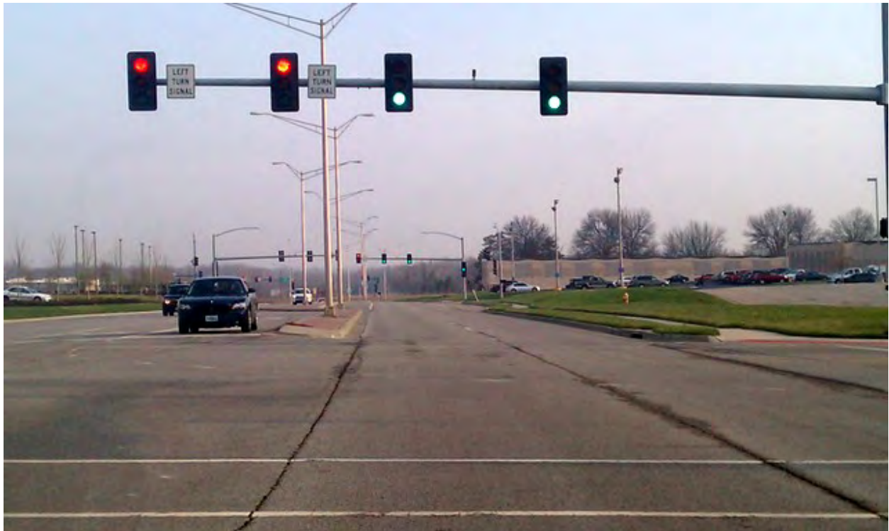
By talking to each other, the traffic signals can intelligently adapt to traffic demand. In this picture, you see several intersections turning green at the same time.
